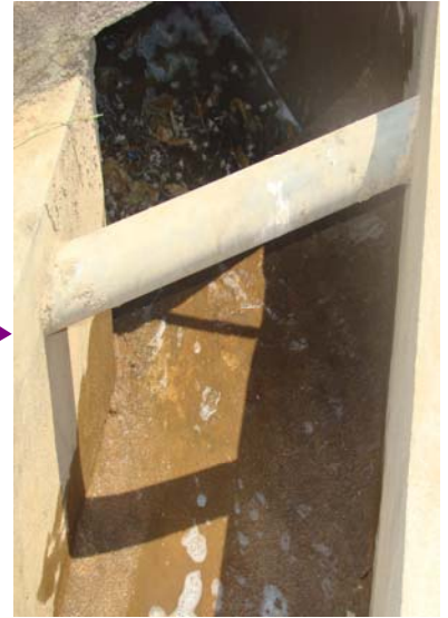
Discharge into Drains
