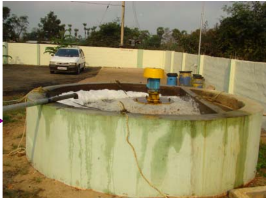
Effluent Treatment Plant
