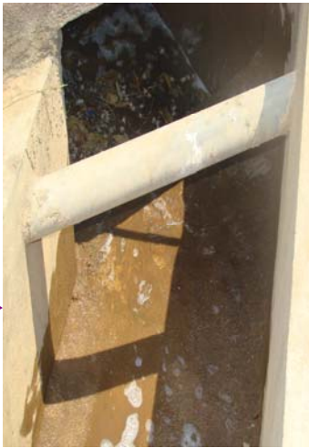
Discharge into Drains
