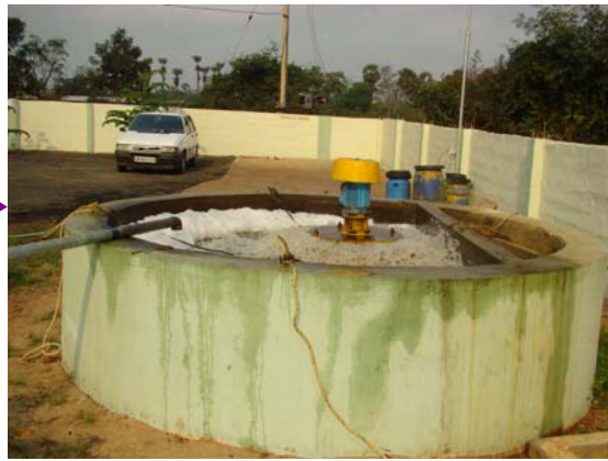
Effluent Treatment Plant
